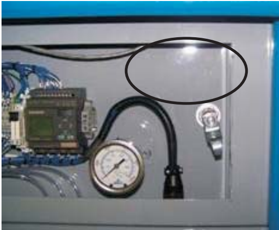
fig. 5.3-2 BAM Upper Control Panel
